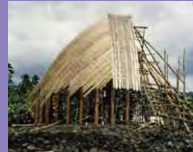
Fale Under Construction Using Traditional Methods, in Asau, Savai'i, August 1978 ©Trustees of the British Museum, Oc,A36.58, AN510422
